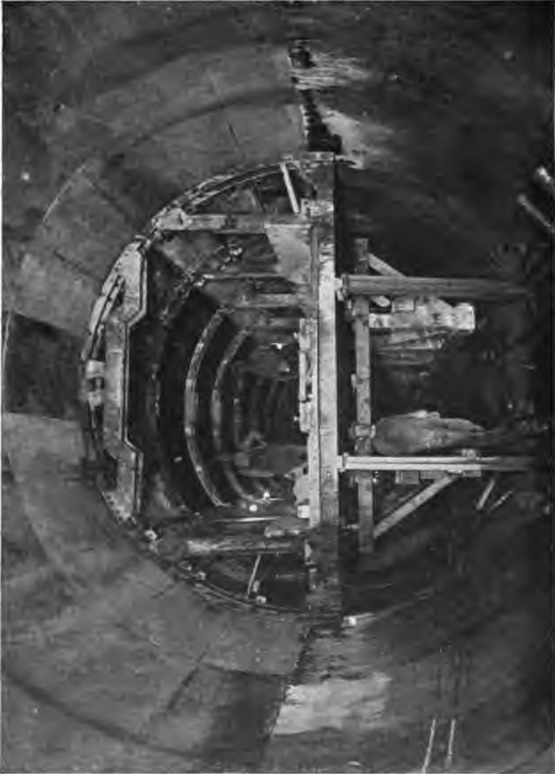
PLATE 102.—Rondout Siphon. Steel Arch Forms and Wooden Carriage for Pressure Tunnel. Carriage runs upon rails—form clears concrete by pulling in sides with turnbuckles and lowering carriage by small screw-jacks.
